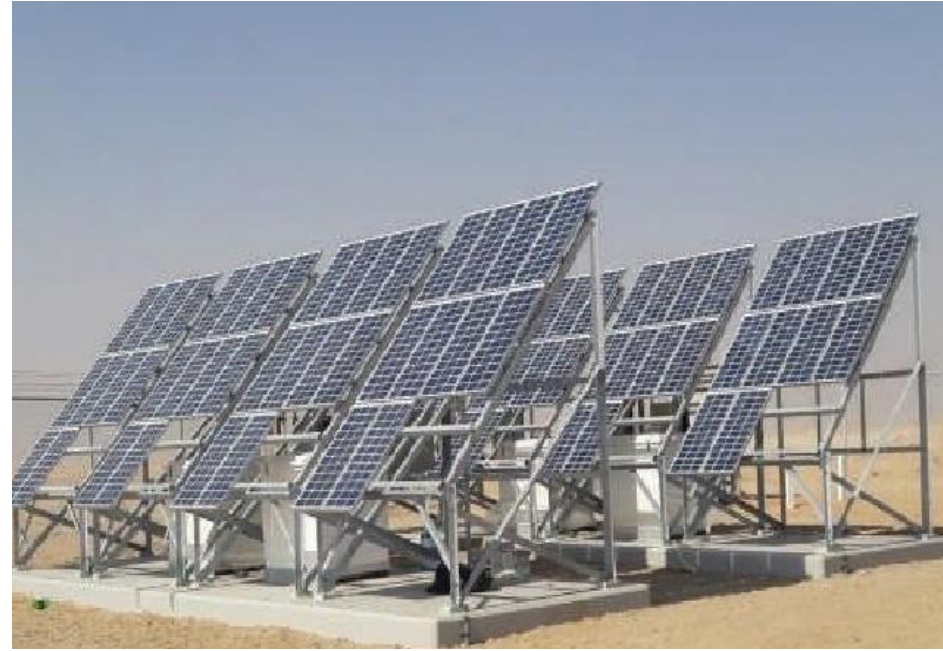
CP Solar Power Supply System
